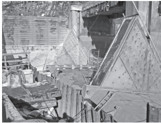
Springbank Dam renovation under way. Note the wall plates welded in place using AGM's spatial location skills to achieve the necessary precision.
